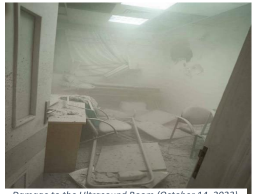
Damage to the Ultrasound Room (October 14, 2023)
